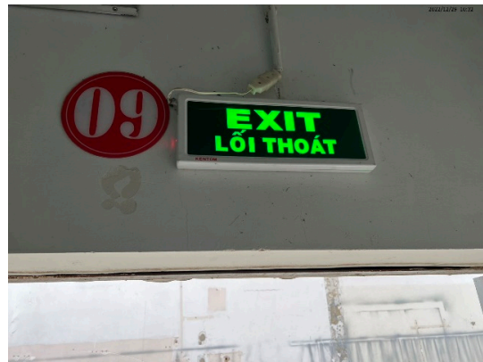
14. Exit sign at door.jpg
