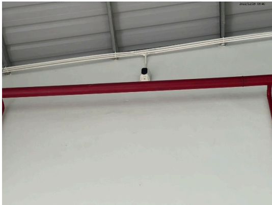
11. Lazer fire alarm system.jpg
